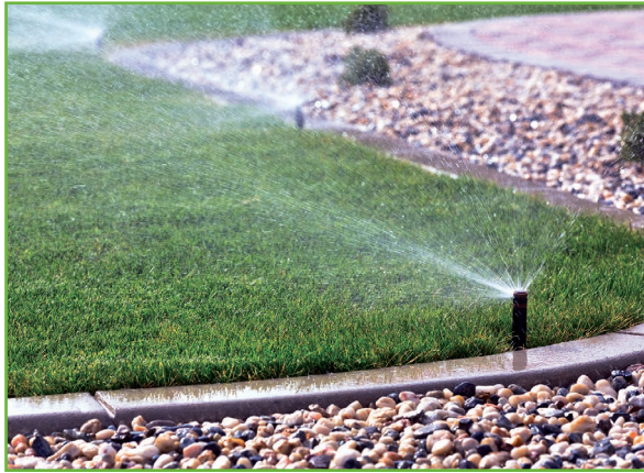
Irrigation systems require backflow prevention devices, which should be tested annually.
