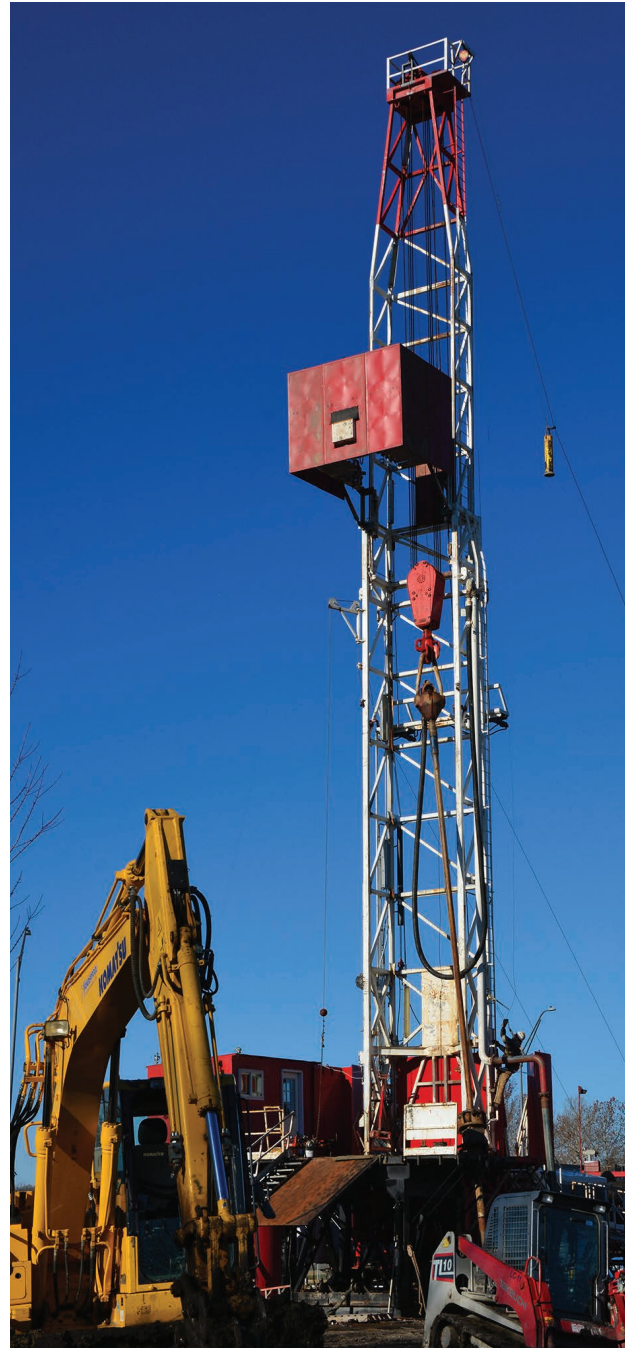
The drilling rig shown above is situated at the southeast corner of Holiday Park.
