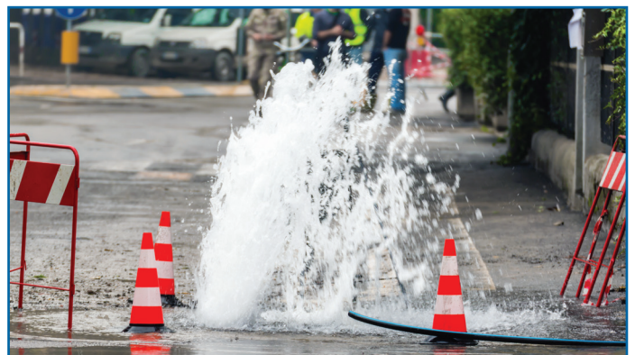
Example of a water main break featured in Folkman's report.
