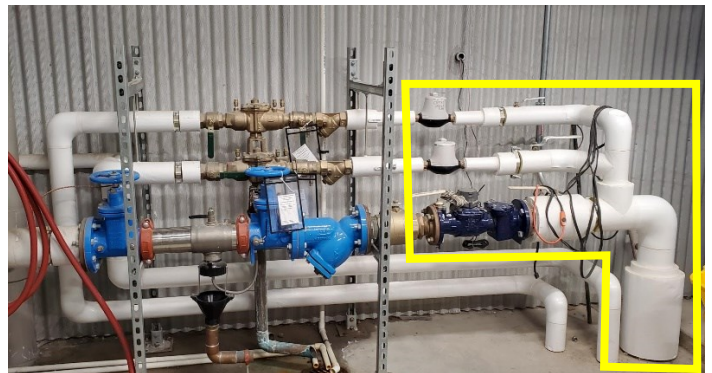
Commercial with Multiple Meters
