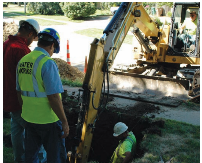
Kevin Trevislyan of the Water Works inspects the replacement progress on 13th Street between Ashworth Road and Pleasant Drive.
